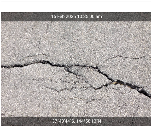
Photo 2: Cracks spreading on Emu Pl.
